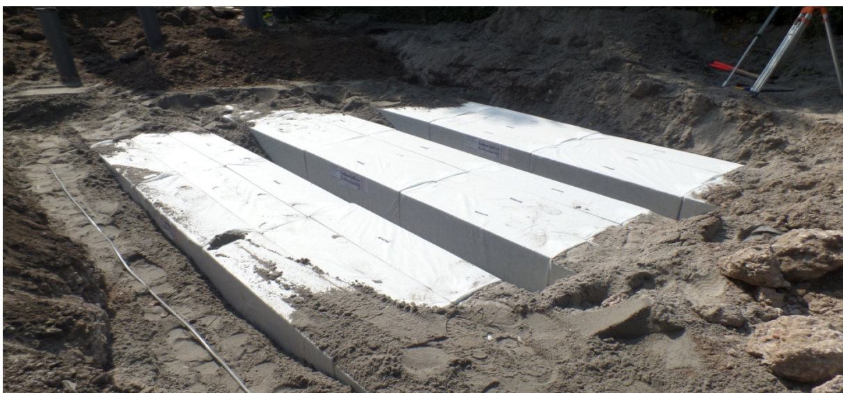
Picture above shows installation of multiple buffers with spacing in between for maximum infiltration capacity.
